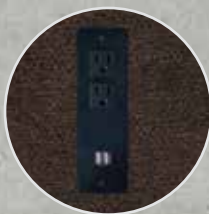
Power outlet in console
